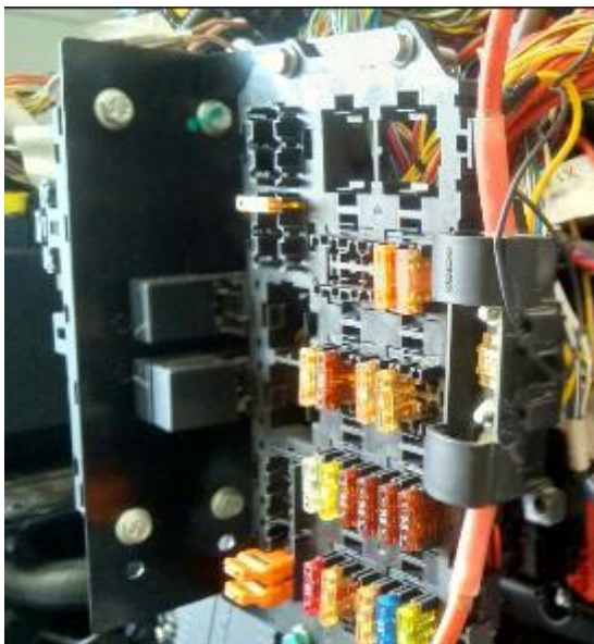
Cabin fuse box
