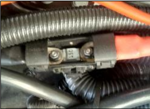
Retarder Power supply fuse (1x150A)
