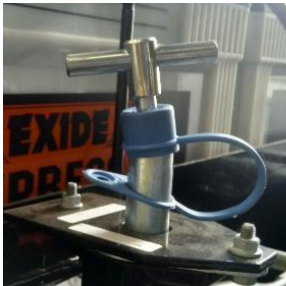
Battery cutoff Switch
